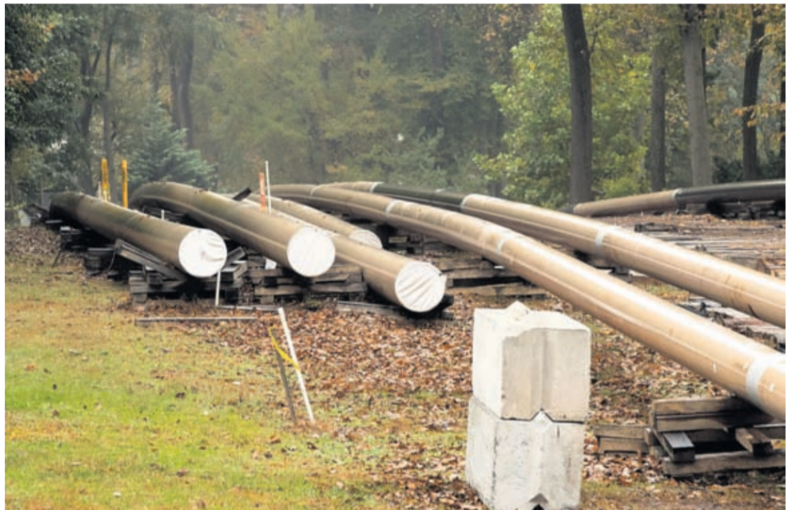
In this Oct. 22, 2019 file photo, pipes lay along a construction site on the Mariner East pipeline in a residential neighborhood in Exton, Pa.
